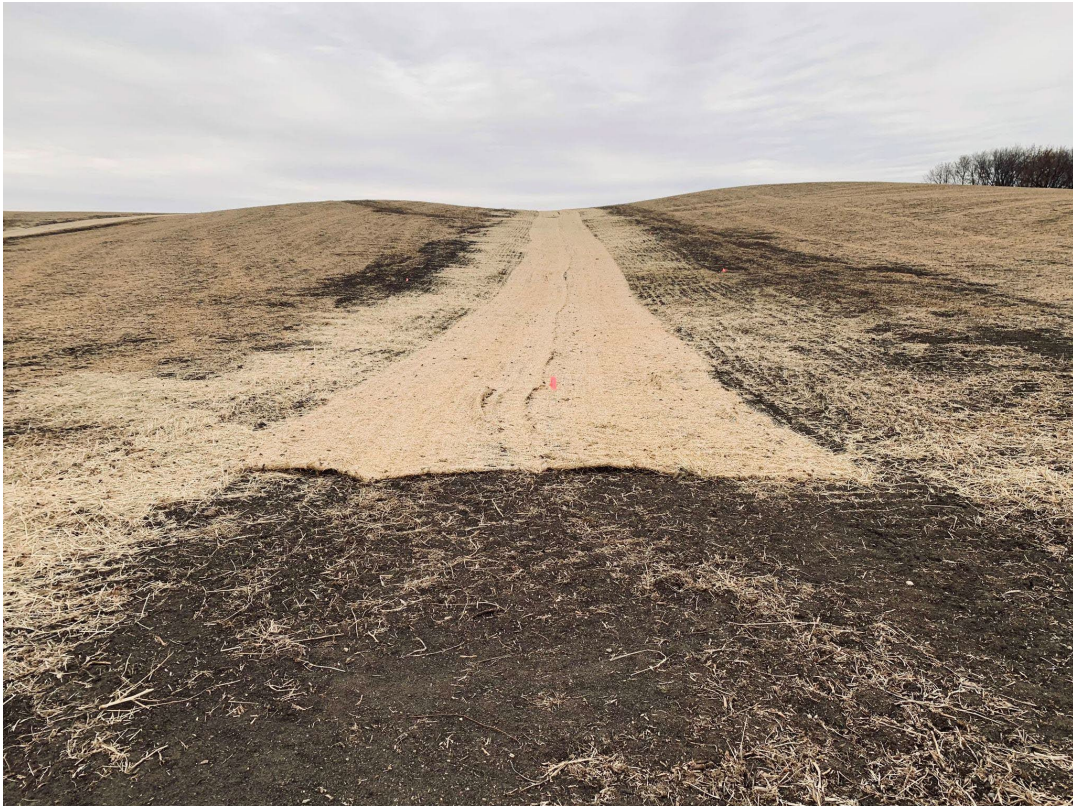
Grassed waterway installation in Watertown Township through the Lake Waconia Subwatershed Assessment Grant..
