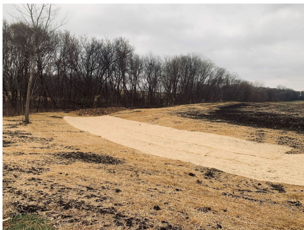
Construction of a grade stabilization and grassed waterway in Dahlgren Township through the SWCD State Cost-share and NRCS EQIP Program..
